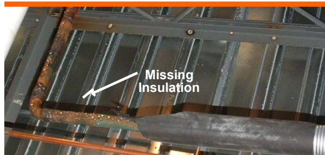
Figure 10 —Missing Suction Line Insulation
